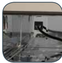
Interior Electrical Outlet
